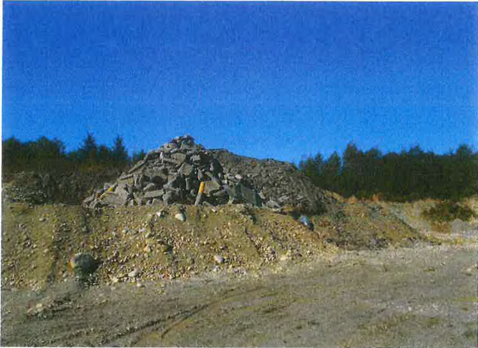
Figure 10. Piles of asphalt and concrete being stored onsite for future crushing and recycling.
