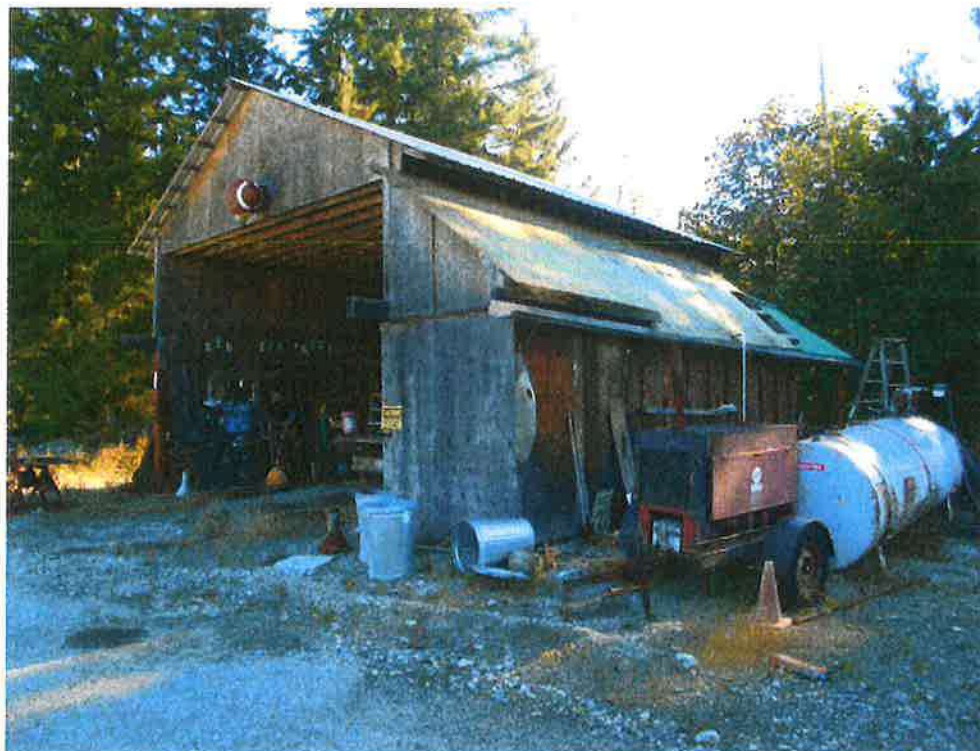
Figure 5. View of the equipment storage and repair building along northeastern property boundary. The 1,000-gallon diesel AST is located along the south side of the building (right side of photo)
